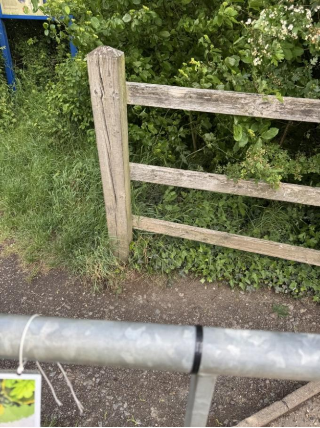
3. The edge of the stile is rotten.
